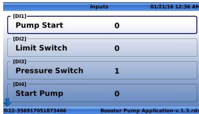
Figure 22: PC-22D Controller, input status.
