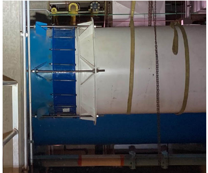
The knife gate valve's narrow face-to-face dimension allowed it to be installed in the confined area.
