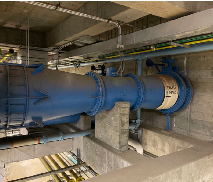
A 48" butterfly valve installed in a filter bypass line was not a good solution for handling the dirty media because of the disc in the center of the flow path.
