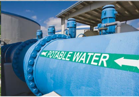
WATER TREATMENT & DISTRIBUTION
