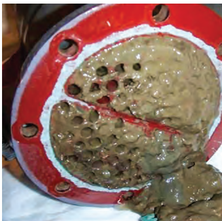
FIG. 1. Heat exchanger tubes fouled with microbes and slime.
