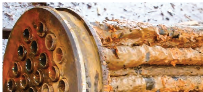
FIG. 1. Fouling and under-deposit corrosion leading to premature bundle replacement.
