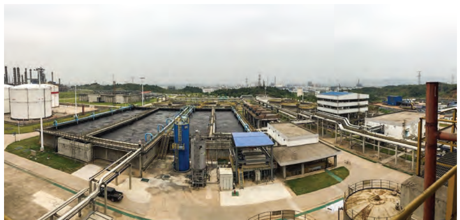
FIG. 1. The refinery's wastewater treatment process units include PACT biological treatment systems and a wet air regeneration (WAR) hydrothermal treatment unit.
