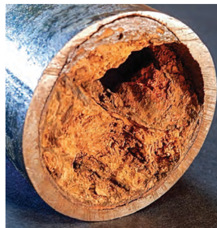
FIG. 2. A pipe nearly blocked by corrosion products.
