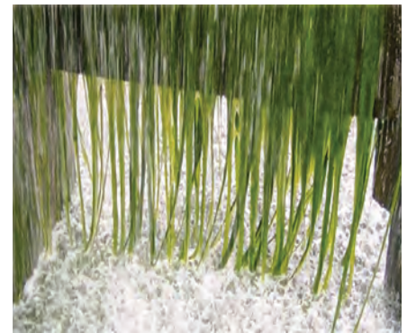
FIG. 4. Severe algae growth in a cooling tower.
