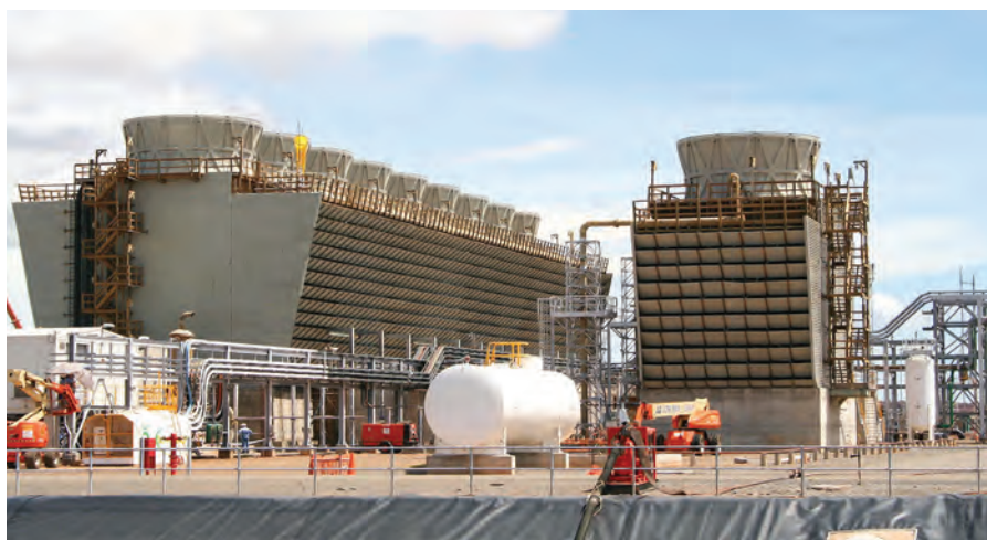
FIG. 1. Cooling towers are often used to transfer heat from processes to the atmosphere, but they have high construction, operational and maintenance costs.
