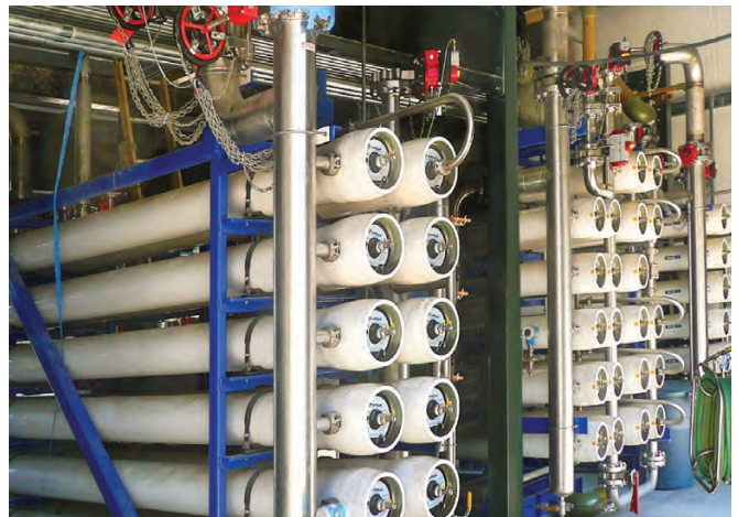
FIG. 3. Membranes (reverse osmosis concentration) can be a water recovery option for HPI/CPI companies. Recommendations are made by water management companies after analysis of operating cost projections, performance needs and feasibility.
