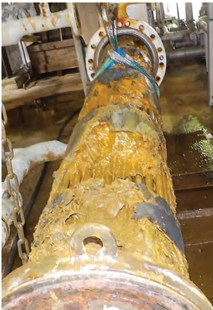
FIG. 3. Closed-loop heat exchanger with dirt.
