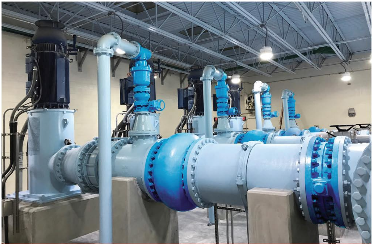
Pump station design with silent check valve installed five pipe diameter lengths from pump discharge.
